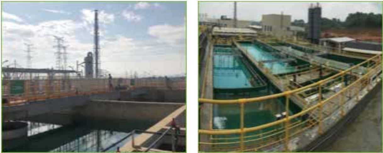
Above: Wastewater Treatment System
