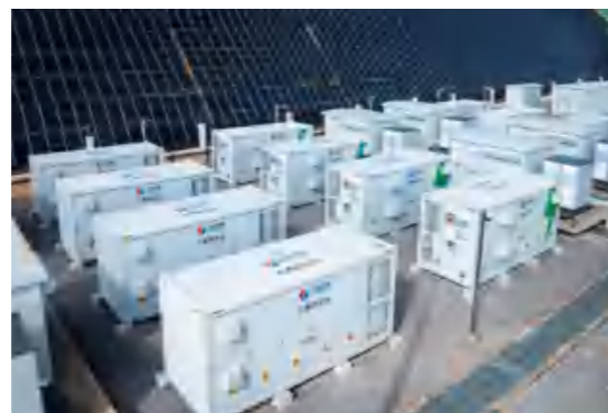
Delivering 42MWh of Energy Storage Systems to the Xiaohelima PV & ESS Project in Yunnan
