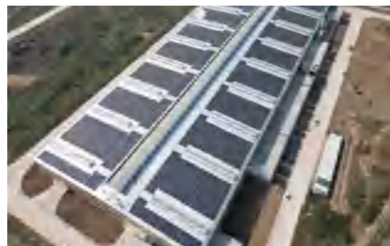
Dongboshengye 2MW rooftop BIPV Project
