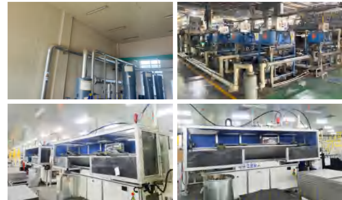
Noise Protection and Improvement Devices
