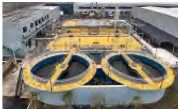
Wastewater Treatment Facilities
