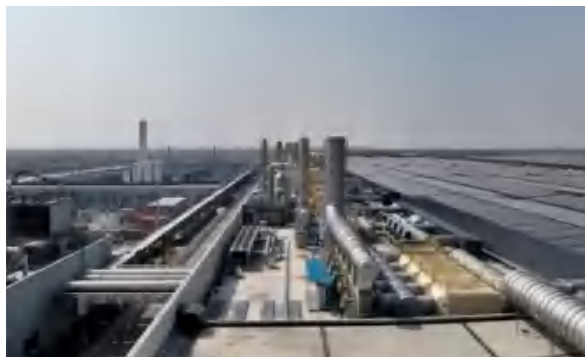
Exhaust Gas Treatment Facilities
